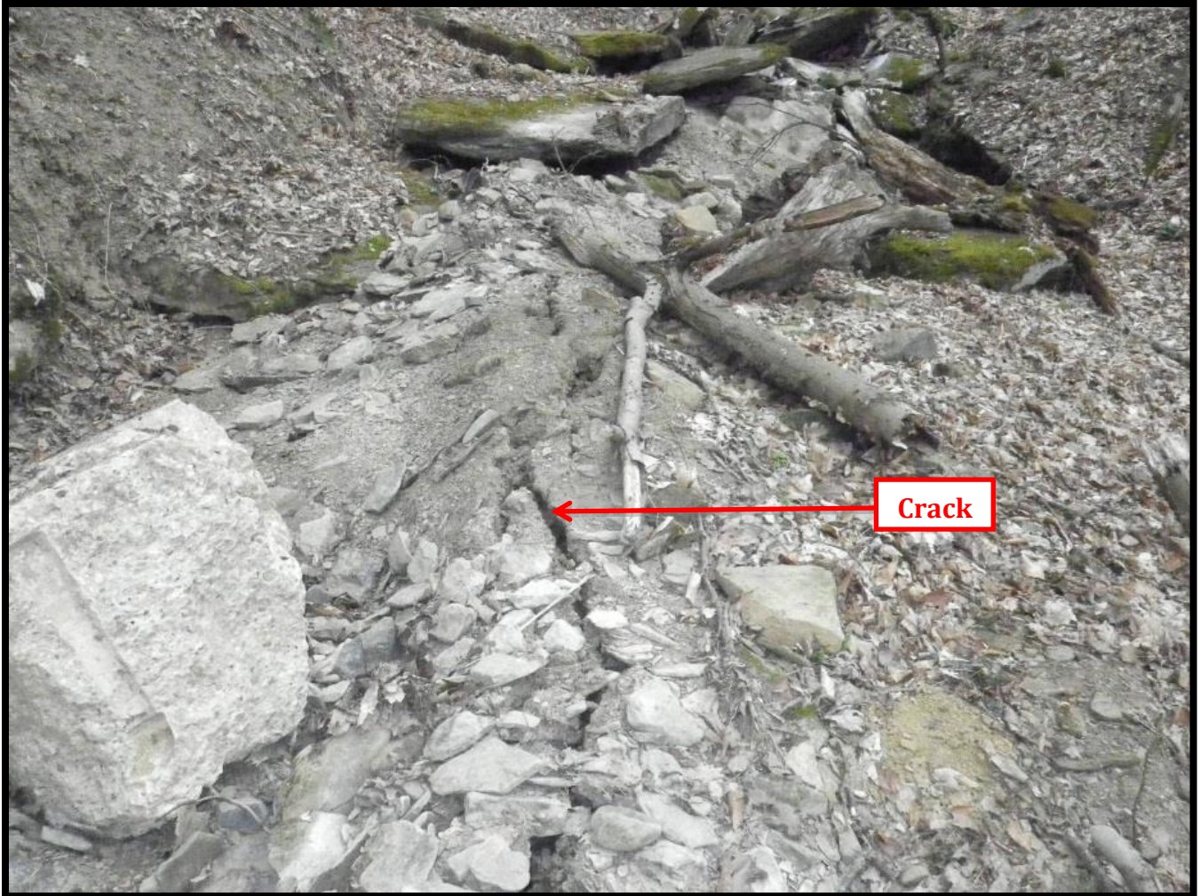
Figure 18. Image showing crack in dewatered streambed coincident with longwall mining. Image courtesy of Steve Ball (WVDEP).
