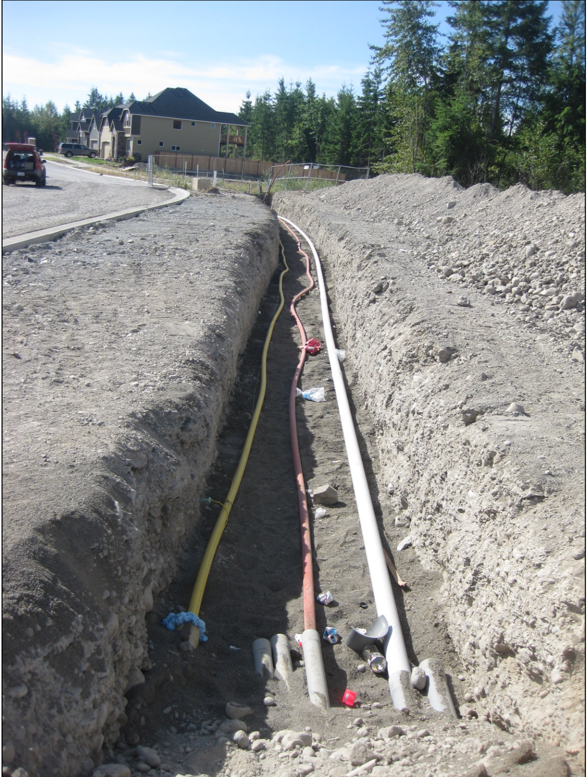
Figure 4 – COLUMBIA VISTA PHASE II TRENCH. Southeast-facing view of the trench along the west side of Overlook Dr. E in the Columbia Vista Phase II housing development (site 1). The trench is excavated in Vashon till (Qvt) with sand fill covering the bottom.
