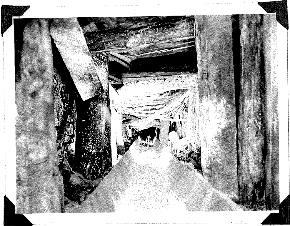
Plate III. Mine 5, 13th East entry, temporary timbering. Note timber breaking from pressure although entry has been driven but 10 days previously through this area; 1640 ft overburden.
